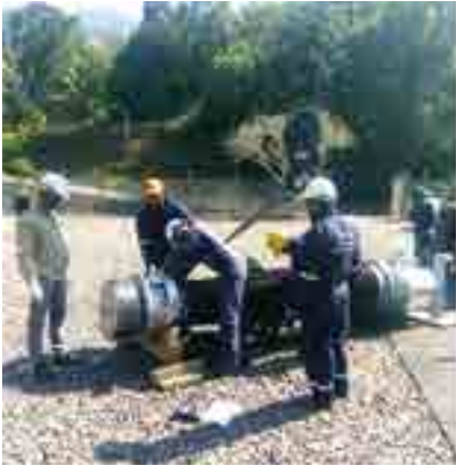
New CT before installation
