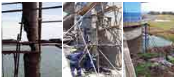
Corroded steel pipe
