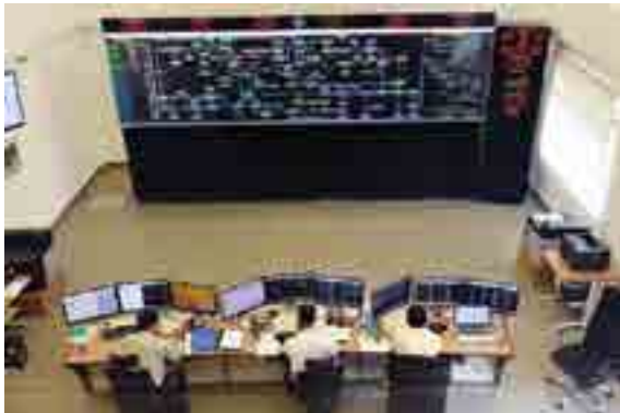
Figure Tr-3: System Control Centre
