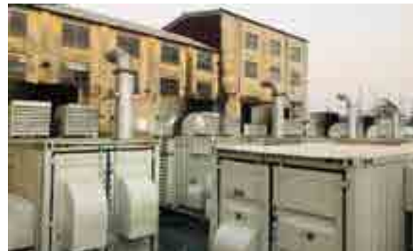
1MW generators at Kolonnawa site -02
