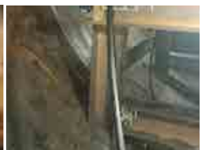
MIV Blade Seal before repair
