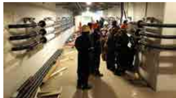
Installation of IPB system at Kukuleganaga Power Plant.
