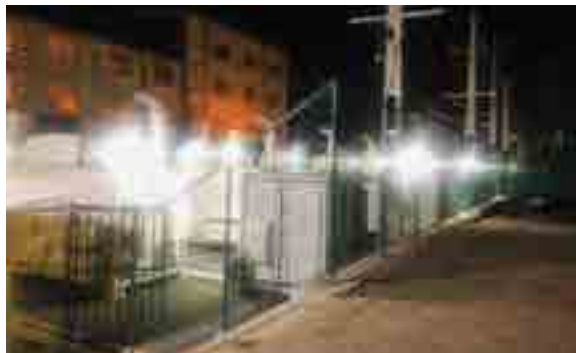
1MW generators at Kolonnawa site -02
