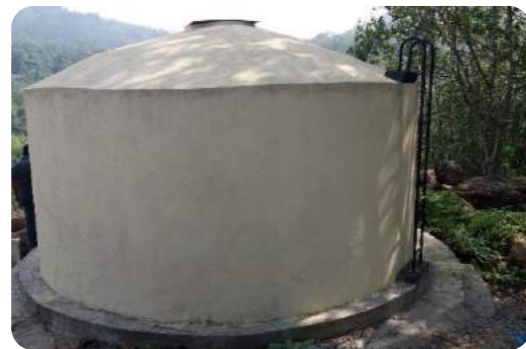
40 c.u.m Ferro Cement Tank at Randew Mawatha CBO
