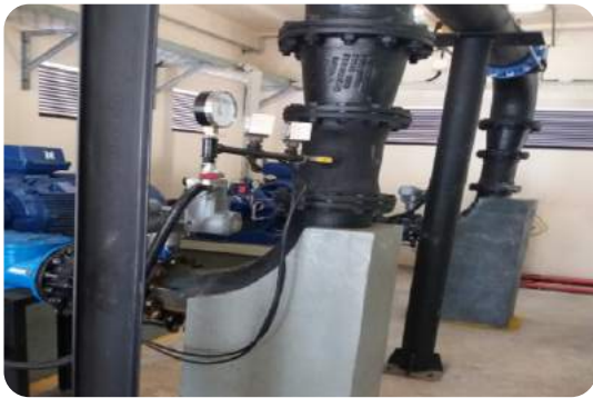
Completed Booster Pumps installation at Keraminiya Booster Pump Station
