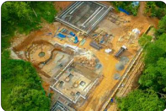
Ukuwela Treatment Plant
