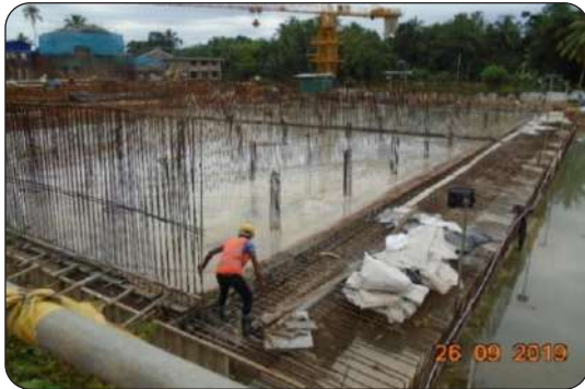
Water Treatment Plant
