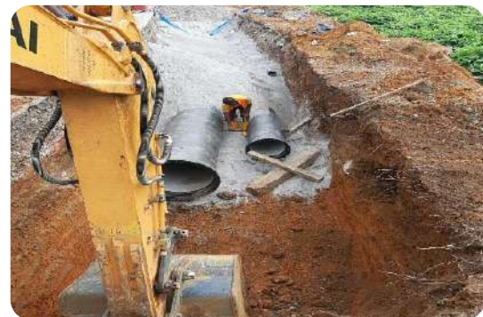
Laying of raw water and clear water pipe lines in one trench
