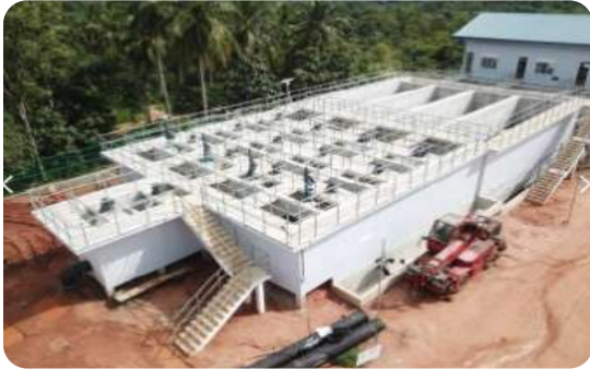
Water Treatment Plant
