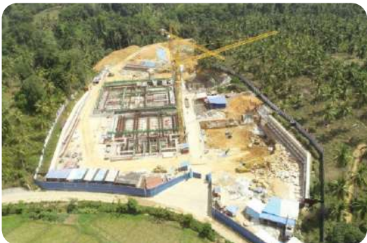
Water Treatment Plant at Karasnagala
