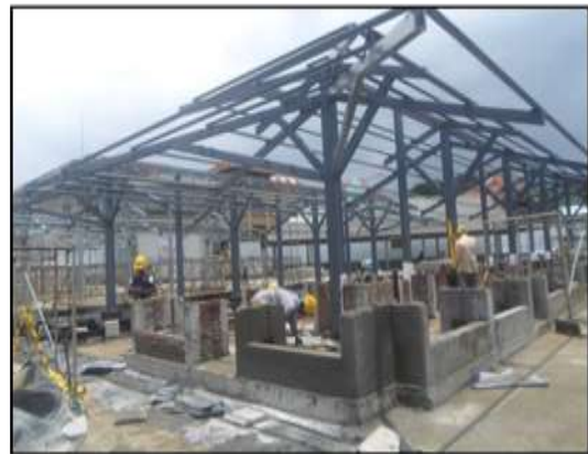
Construction of Urban Council Carpark under the Kandy, Strategic City Development Project
