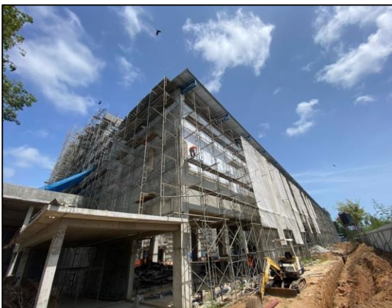
Construction of Import Cargo Terminal building at the Bandaranayke International Air Port (BIA), Katunayaka, Stage I
